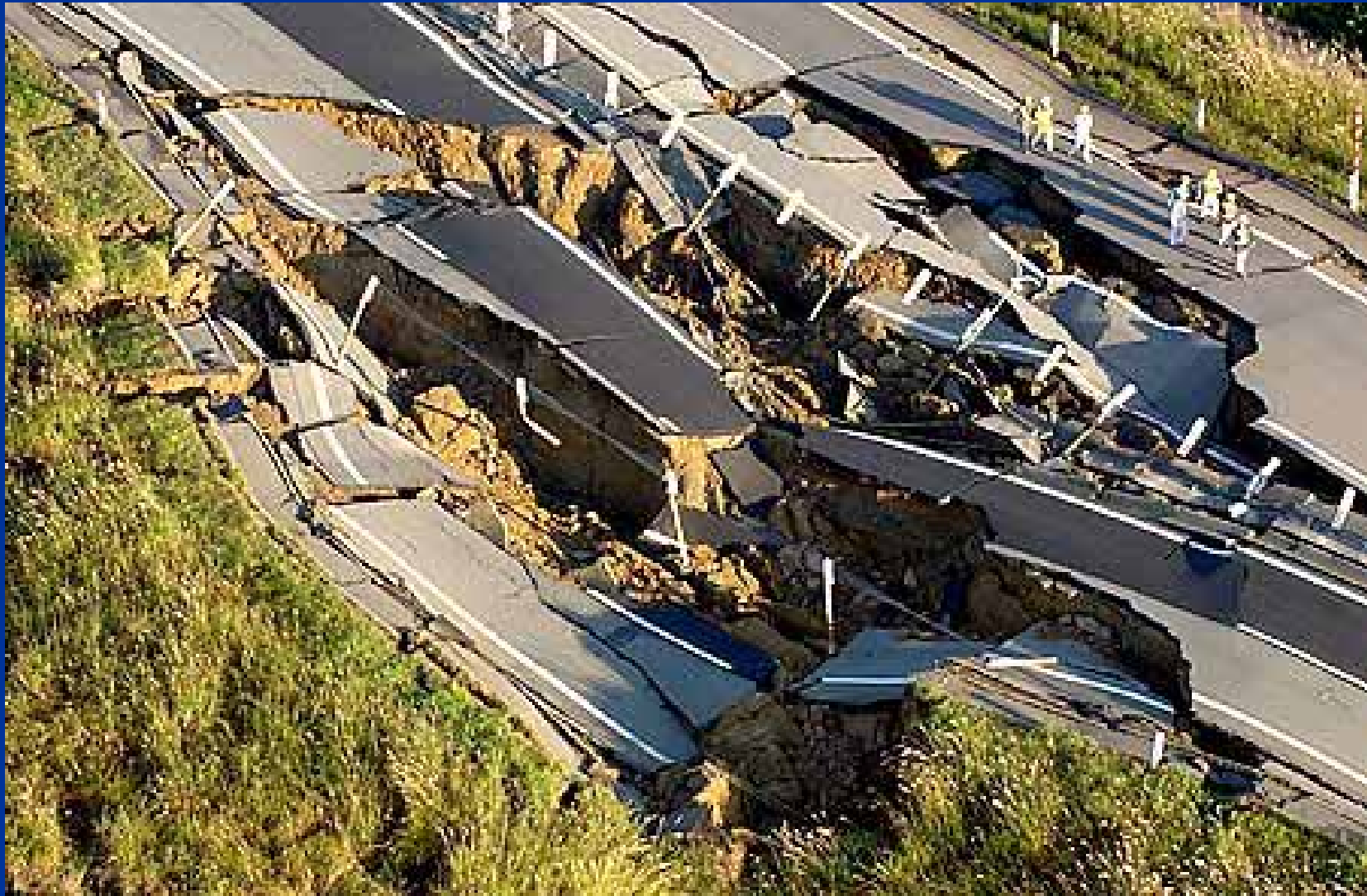
Collapse of Kanetsu Highway
